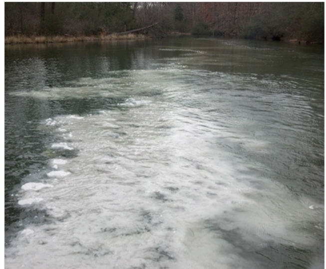
Figure 7. Lime is washed from a barge using a high-pressure hose and is thoroughly mixed throughout the pond.
